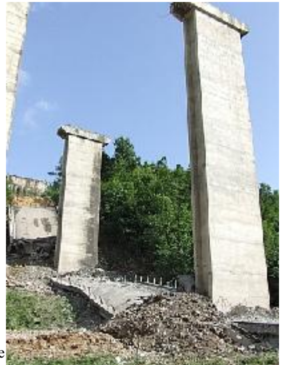
Figure 3: example of viaduct demolition where pylons were left in place to support the new weathering-steel (COR_TEN) continuous deck replacing the reinforced concrete one being demolished.
