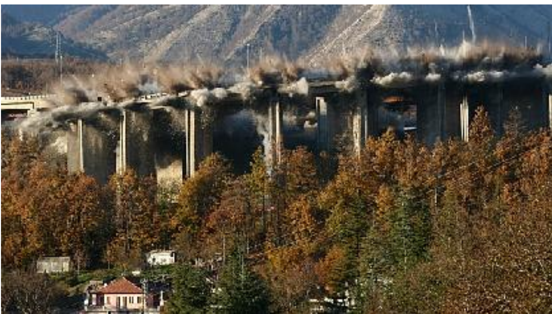
Figure 4: decks cut down in the proximity of a residential quarter.
