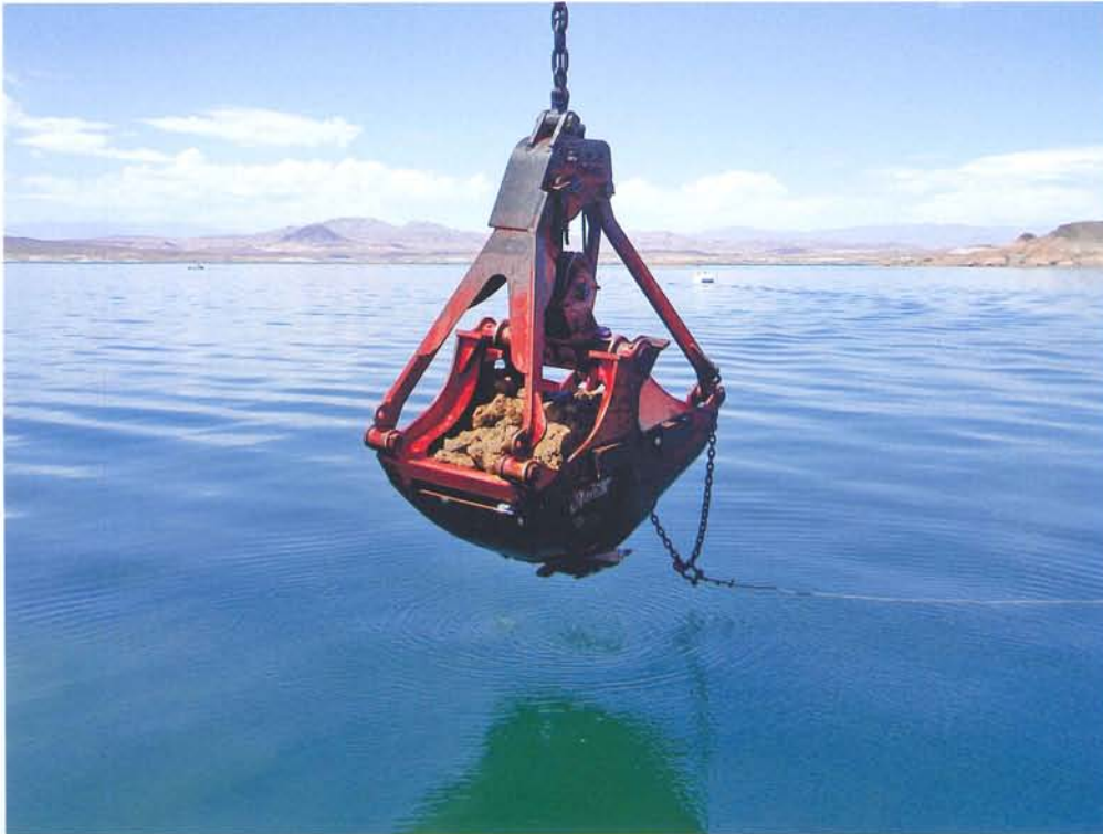
FIGURE 4.19 Nearly all of the debris created by the shaped charges, more than 33,000 yd 3 [25,230 m 3 ], was removed by crane and clamshell bucket operations.
